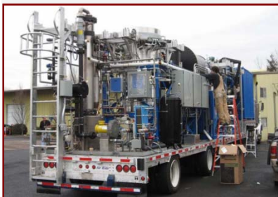
Mobile PEM™ plasma arc plant, courtesy of InEnTec.
