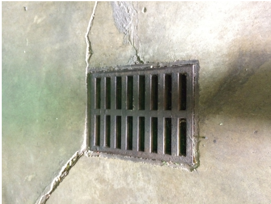
Photo #4: Cracks in concrete floor in main shop
