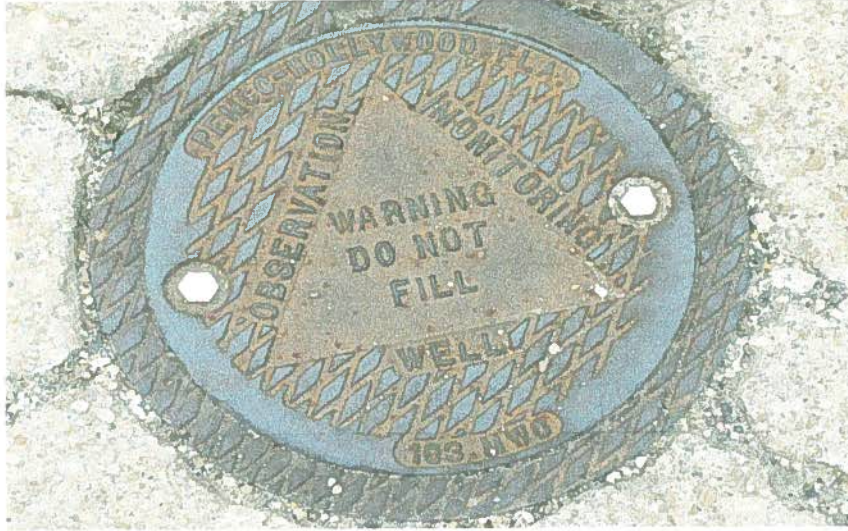
Ground Water Monitoring Well
