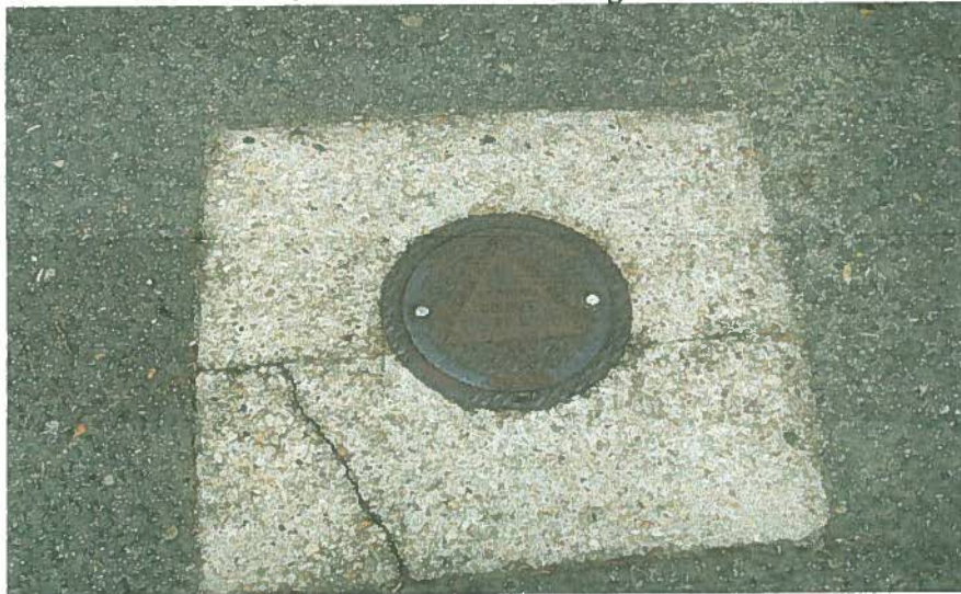
Ground Water Monitoring Well
