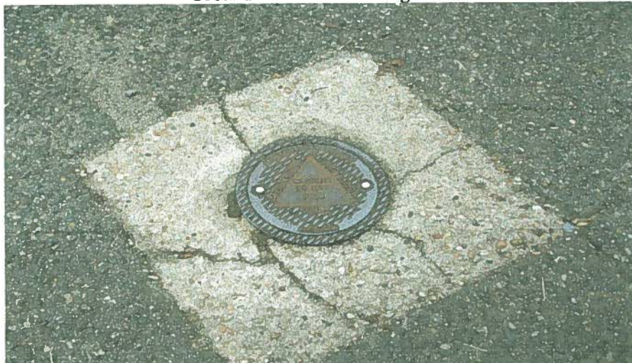
Ground Water Monitoring Well
