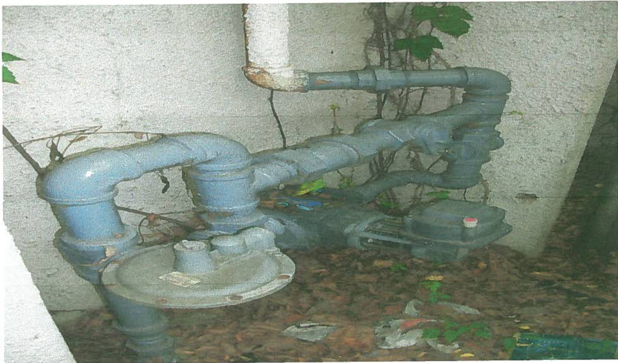
Natural Gas Line
