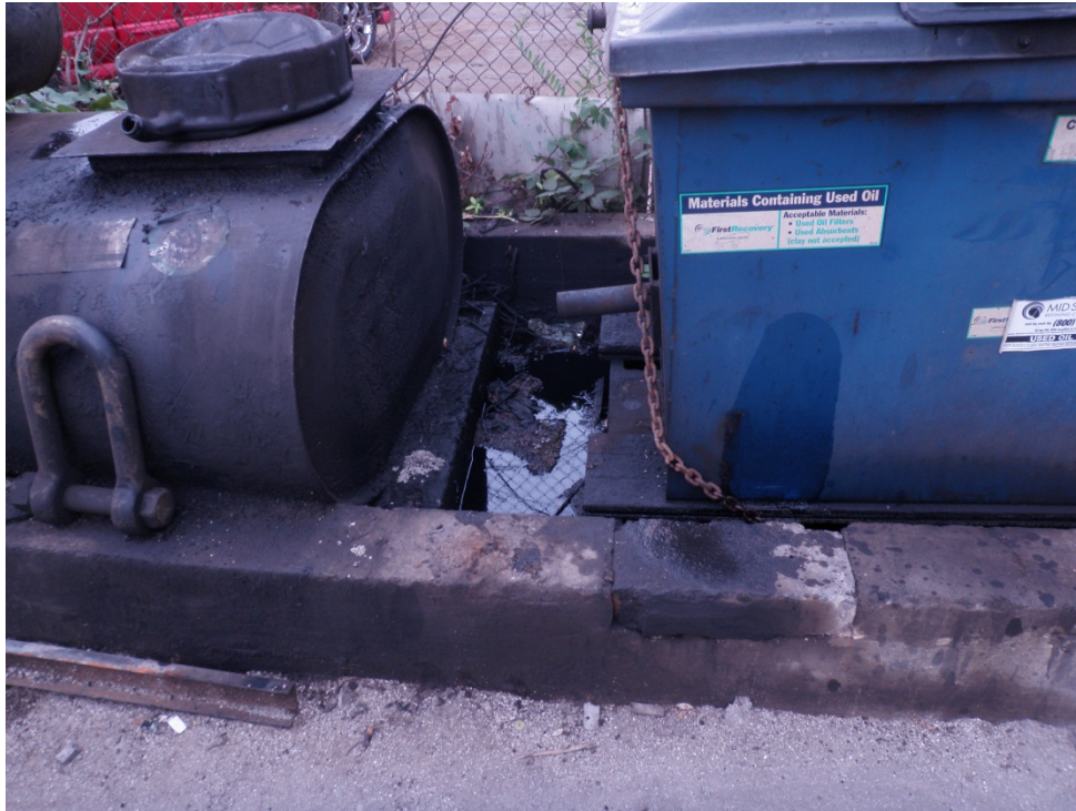
Photo #3: Oil located in AST secondary containment in southeastern portion of Square 0605, Lot 0802
