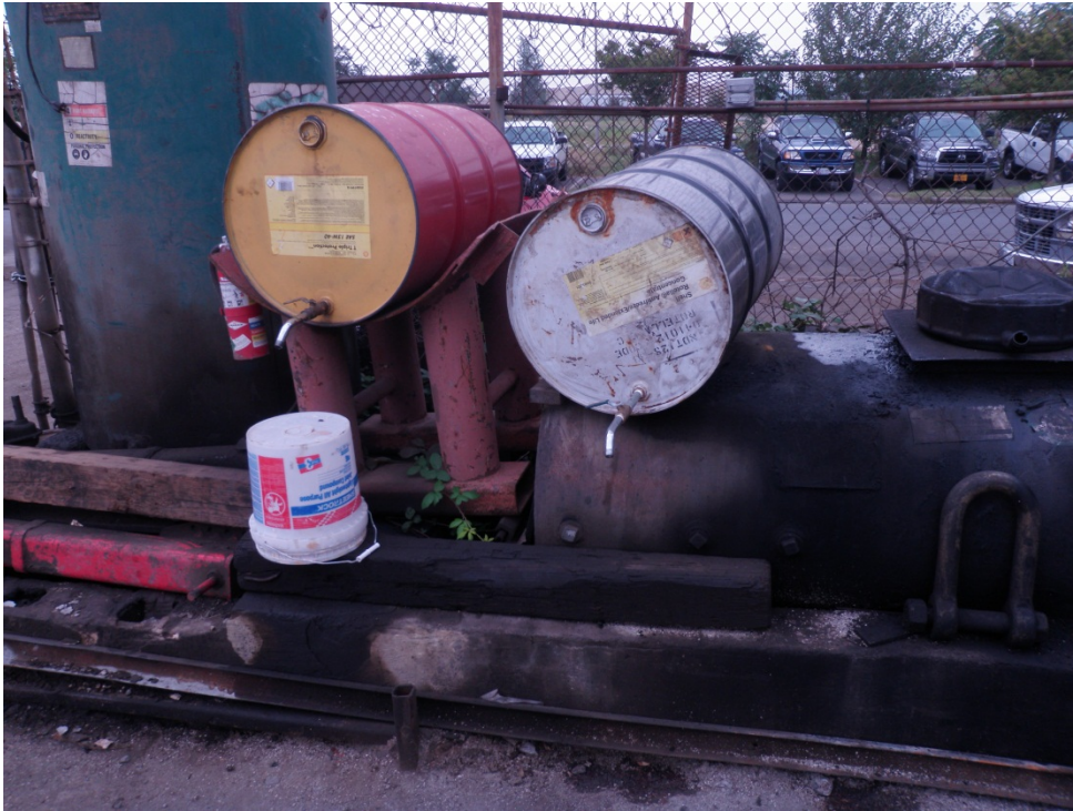
Photo #1: View from the west of ASTs in southeastern portion of Square 0605, Lot 0802
